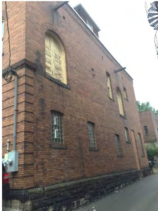
Photograph 22. Pittsburgh EMS Station, Culloden Way Facade, Facing Southeast. Source: Calvin A Yoder.
