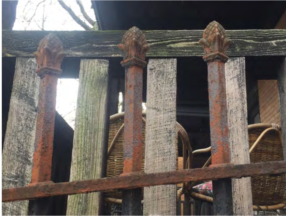
Photograph 21. Pittsburgh EMS Station, Southern Fence Detail, Facing South. Source: Calvin A Yoder.
