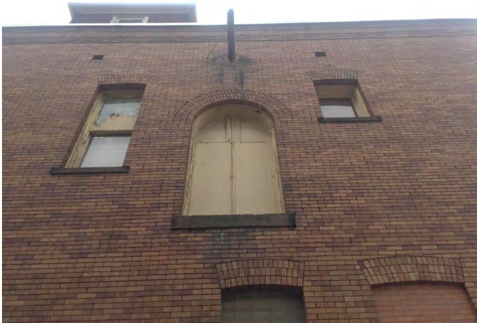
Photograph 25. Pittsburgh EMS Station, Culloden Way Facade, Southern Hayloft, Facing Northeast. Source: Calvin A Yoder.
