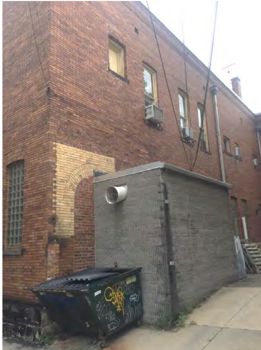
Photograph 18. Pittsburgh EMS Station, Southern Facade, Gas Storage Addition, Facing Northeast. Source: Calvin A Yoder.
