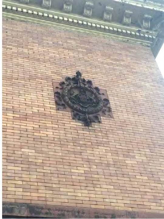
Photograph 9. Pittsburgh EMS Station, Filbert Street Facade, Northern Crest Relief, Facing West. Source: Calvin A Yoder.
