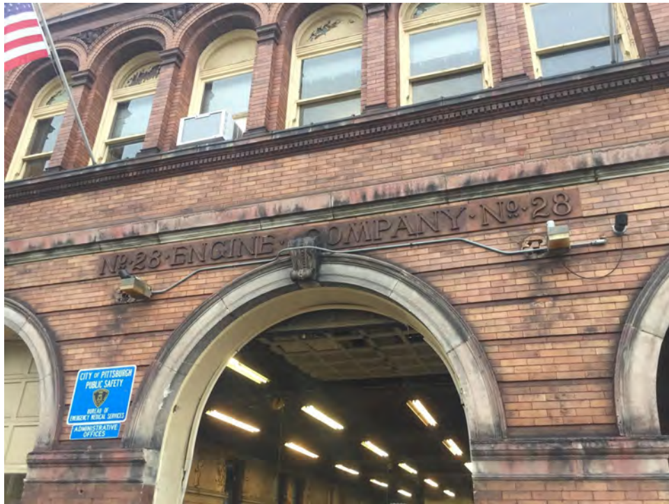
Photograph 5. Pittsburgh EMS Station, Filbert Street Facade, Center Bay Detail, Facing South. Source: Calvin A Yoder.
