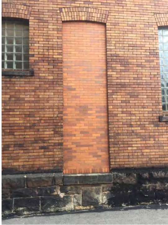
Photograph 23. Pittsburgh EMS Station, Culloden Way Facade, Alteration Detail, Facing East. Source: Calvin A Yoder.
