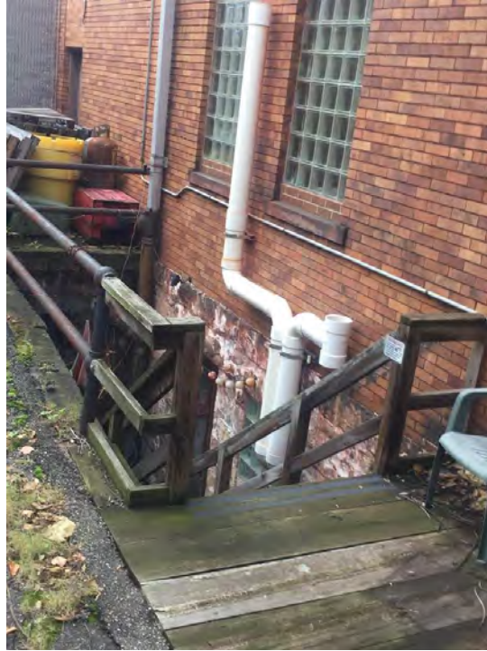
Photograph 19. Pittsburgh EMS Station, Filbert Street Facade, Basement Entrance, Facing West. Source: Calvin A Yoder.
