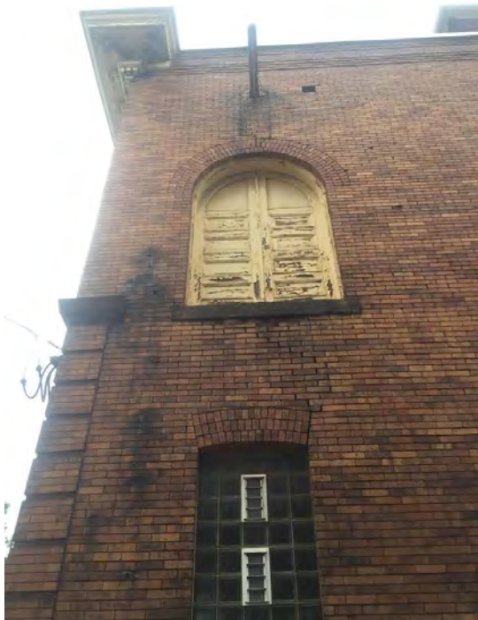
Photograph 24. Pittsburgh EMS Station, Culloden Way Facade, Northern Hayloft, Facing Northeast. Source: Calvin A Yoder.
