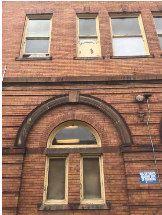
Photograph 12. Pittsburgh EMS Station, Elmer Street Facade, Fenestration Detail, Facing Southeast. Source: Calvin A Yoder.
