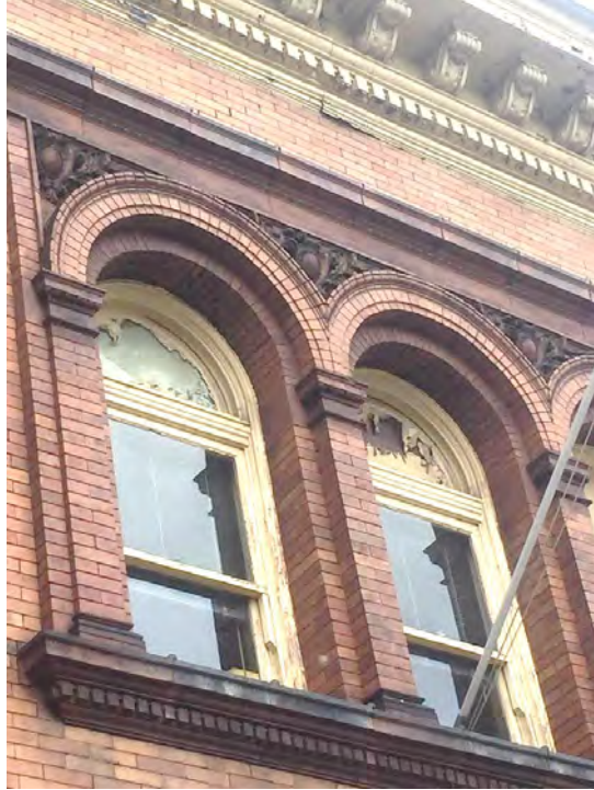
Photograph 7. Pittsburgh EMS Station, Filbert Street Facade, Second Story Arcading Detail, Facing West. Source: Calvin A Yoder.
