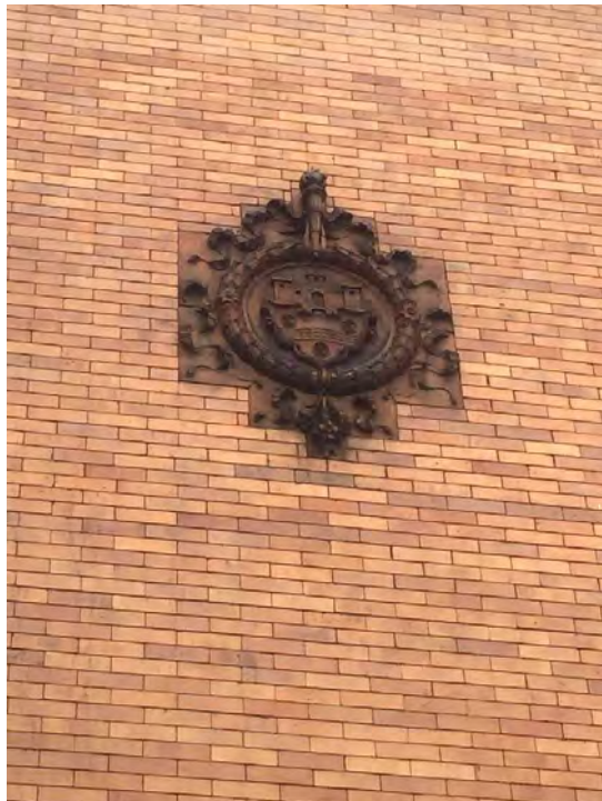
Photograph 8. Pittsburgh EMS Station, Filbert Street Facade, Southern Crest Relief, Facing West. Source: Calvin A Yoder.
