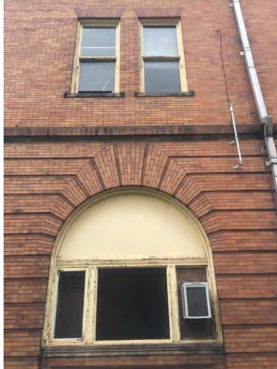
Photograph 11. Pittsburgh EMS Station, Elmer Street Facade, East Fenestration, Facing Southeast. Source: Calvin A Yoder.
