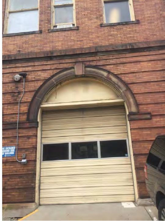
Photograph 13. Pittsburgh EMS Station, Elmer Street Facade, Easternmost Portal, Facing Southeast. Source: Calvin A Yoder.
