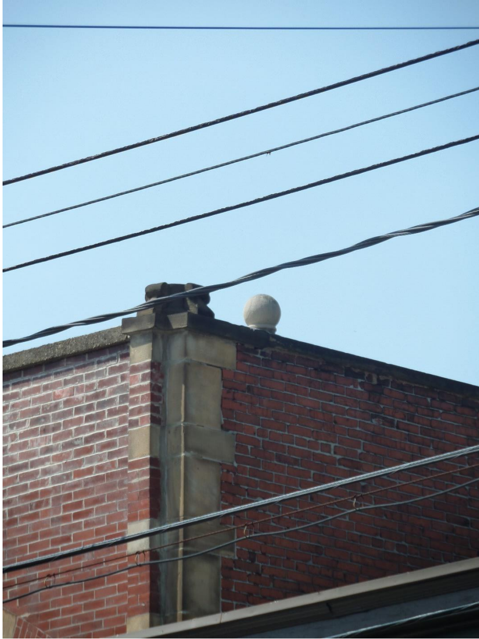
Photo. 8. Former Carrick Municipal Building, Parapet Corner Column and Stone Finial, Brownsville Road Façade, May 15, 2018. Source: Antonio Parente.
