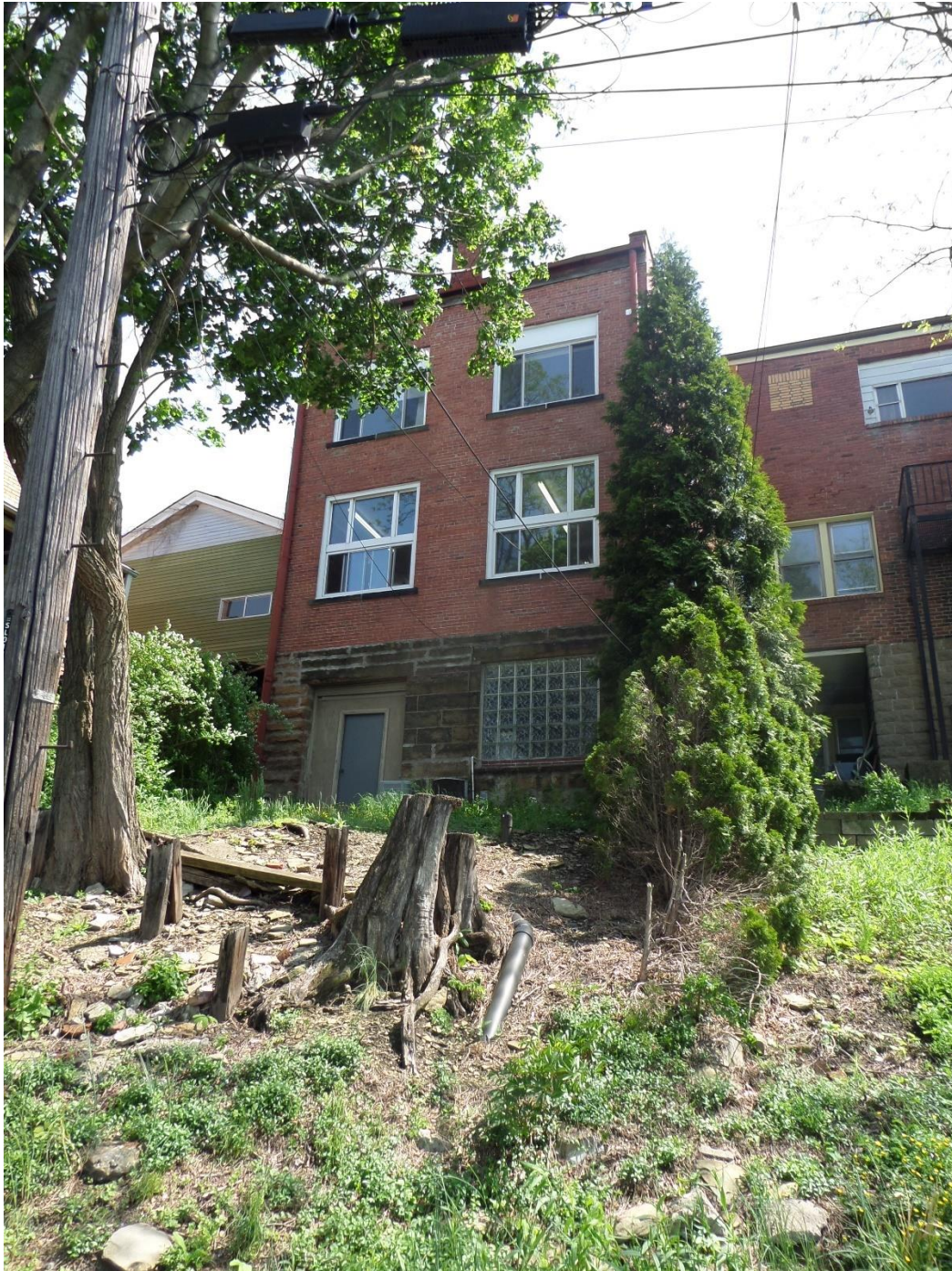
Photo. 9. Former Carrick Municipal Building, Dellrose Street Façade and Hillside , May 15, 2018. Source: Antonio Parente.
