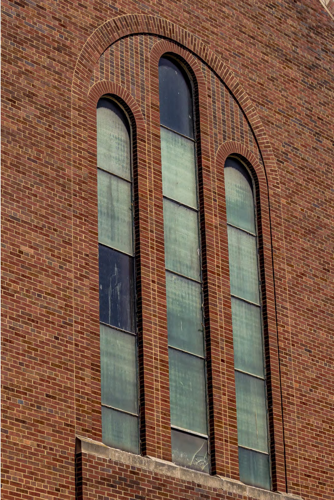
Photo. 4. Former Holy Family Church, Transept Windows , June, 2018. Source: Preservation Pittsburgh.
