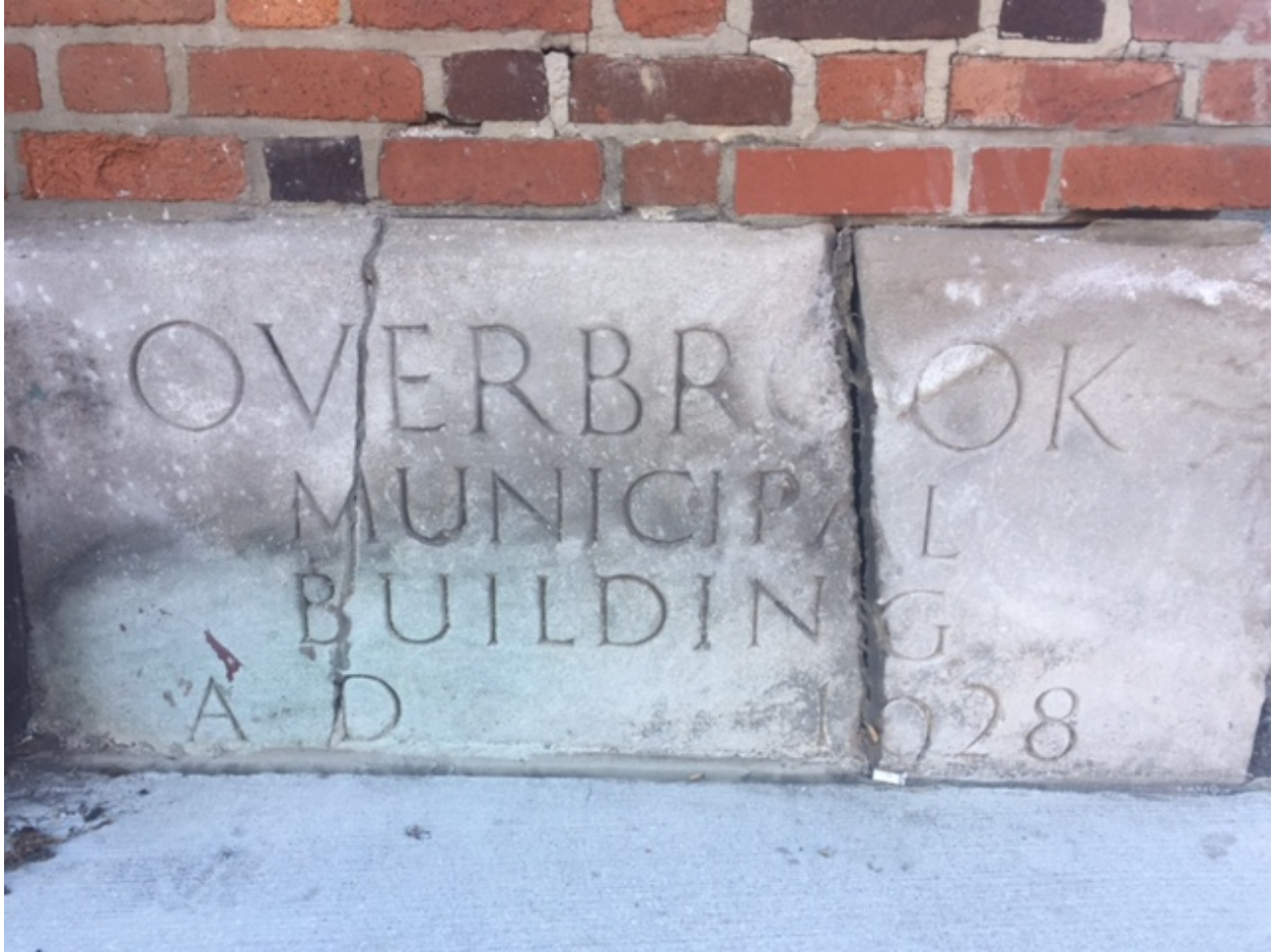
Photo. 6. Overbrook Municipal Building Cornerstone, Former Overbrook Municipal Building, Saw Mill Run Boulevard Façade, March 2, 2017. Source: Matthew W.C. Falcone.
