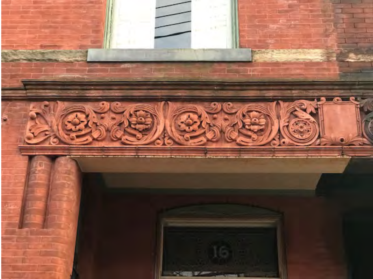
Photo. 3. 417 Lockhart Street, Primary Façade, scroll engraving & transom stained glass with original house numbering. December, 2019. Source: Matthew W.C. Falcone.
