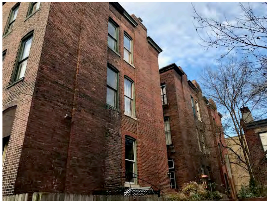
Photo. 6. 417 Lockhart Street, Rear of structure from Moravian Way. December, 2019. Source: Matthew W.C. Falcone.
