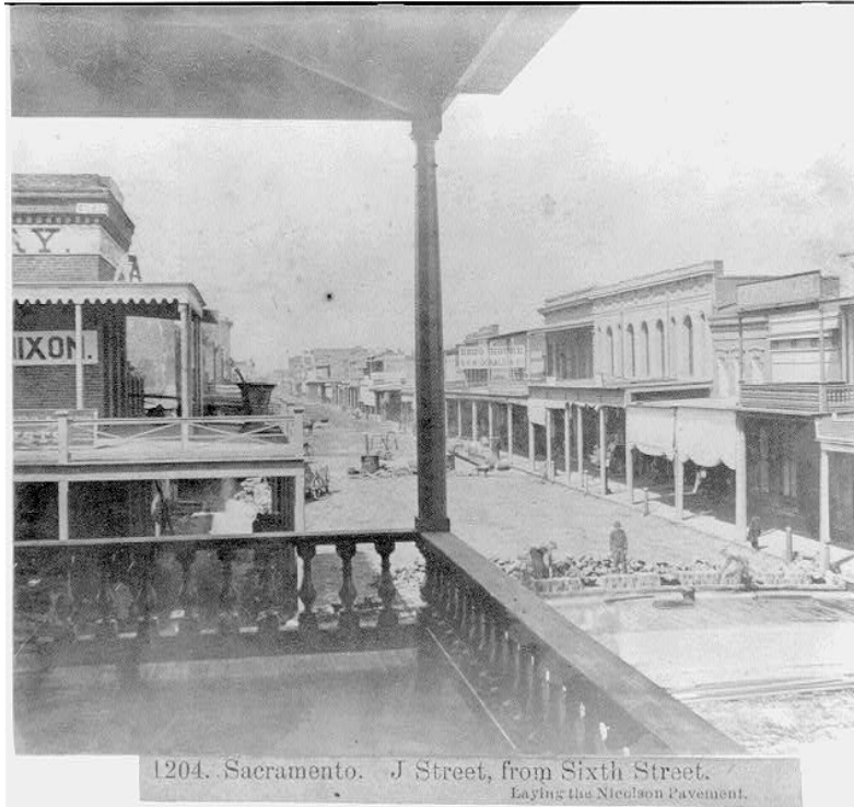
Fig. 26. Sacramento, J Street from Sixth Street, Laying of the Nicolson Pavement, Source: http://cdn.loc.gov/service/pnp/cph/3a20000/3a28000/3a28000/3a28030r.jpg (accessed on September 14, 2016).
