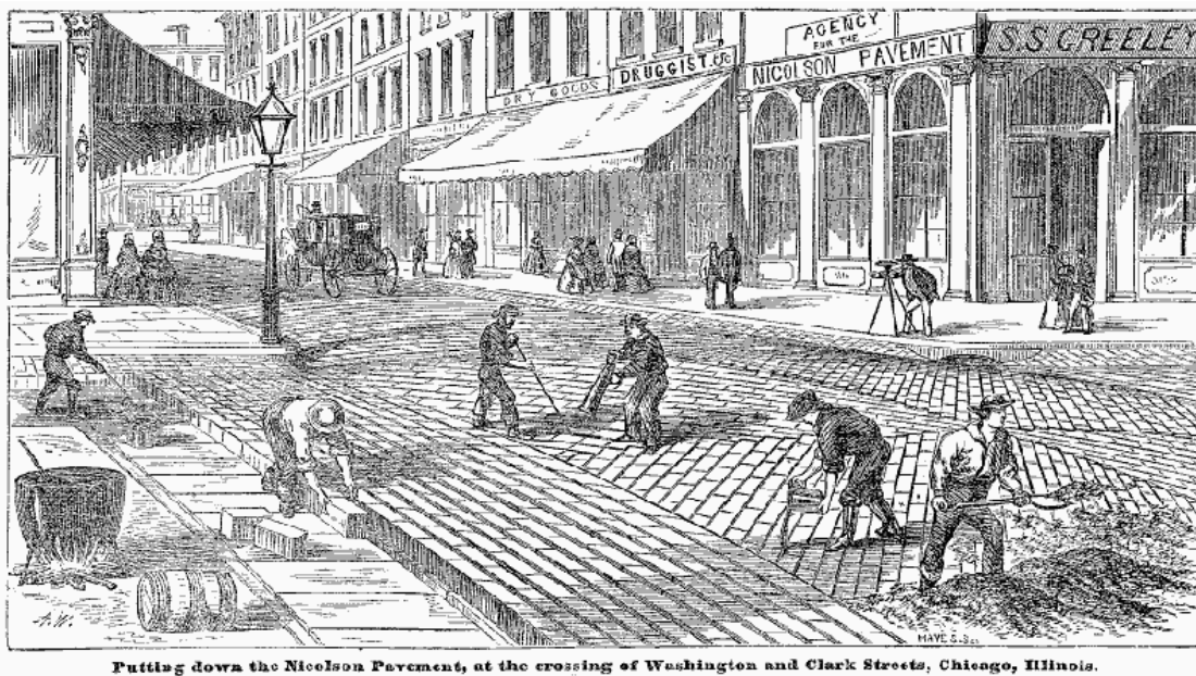
Fig. 27. Putting Down the Nicolson Pavement, at the Crossing of Washington and Clark Streets, Chicago, Illinois. Source: http://www.urbanremainschicago.com/wordpress/wp-content/uploads/2014/11/nicolson_pavement.gif (accessed on September 14, 2016).
