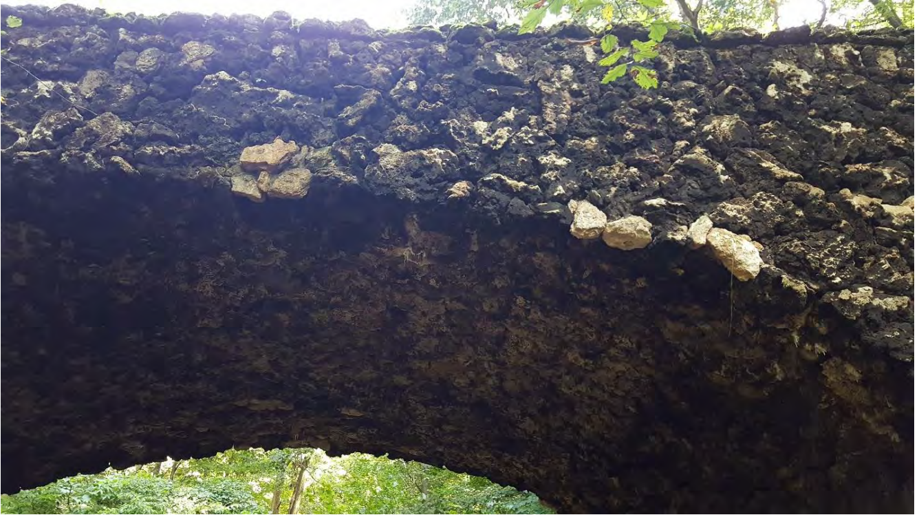
Fig. 25. Black underside of Upper Run Bridge, September 10, 2016, Source: Alayna Jordan.
