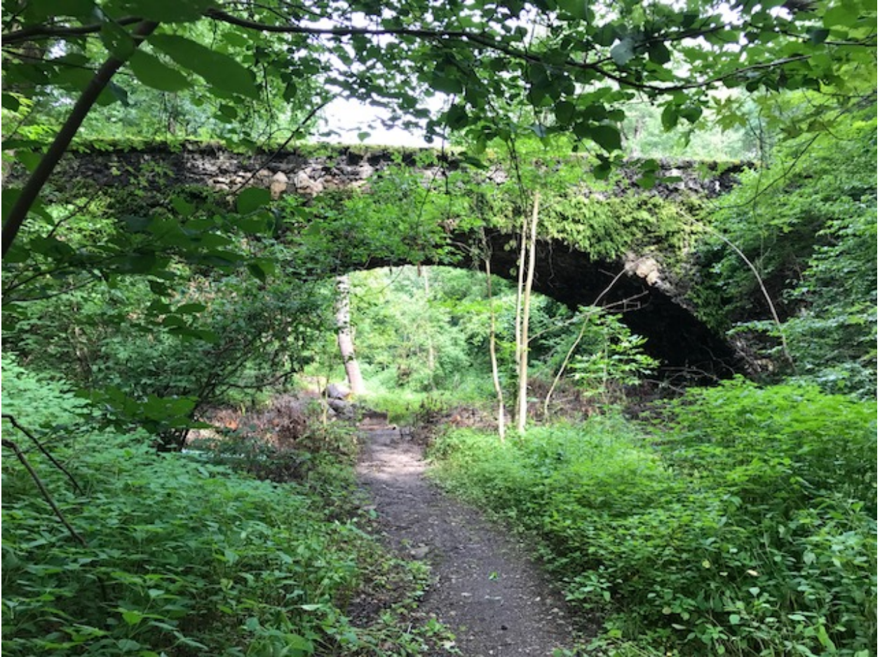
Photo 8. Tufa Bridge II (Elliptical Arch) . Schenley Park, June 2, 2017. Source: Matthew W.C. Falcone.
