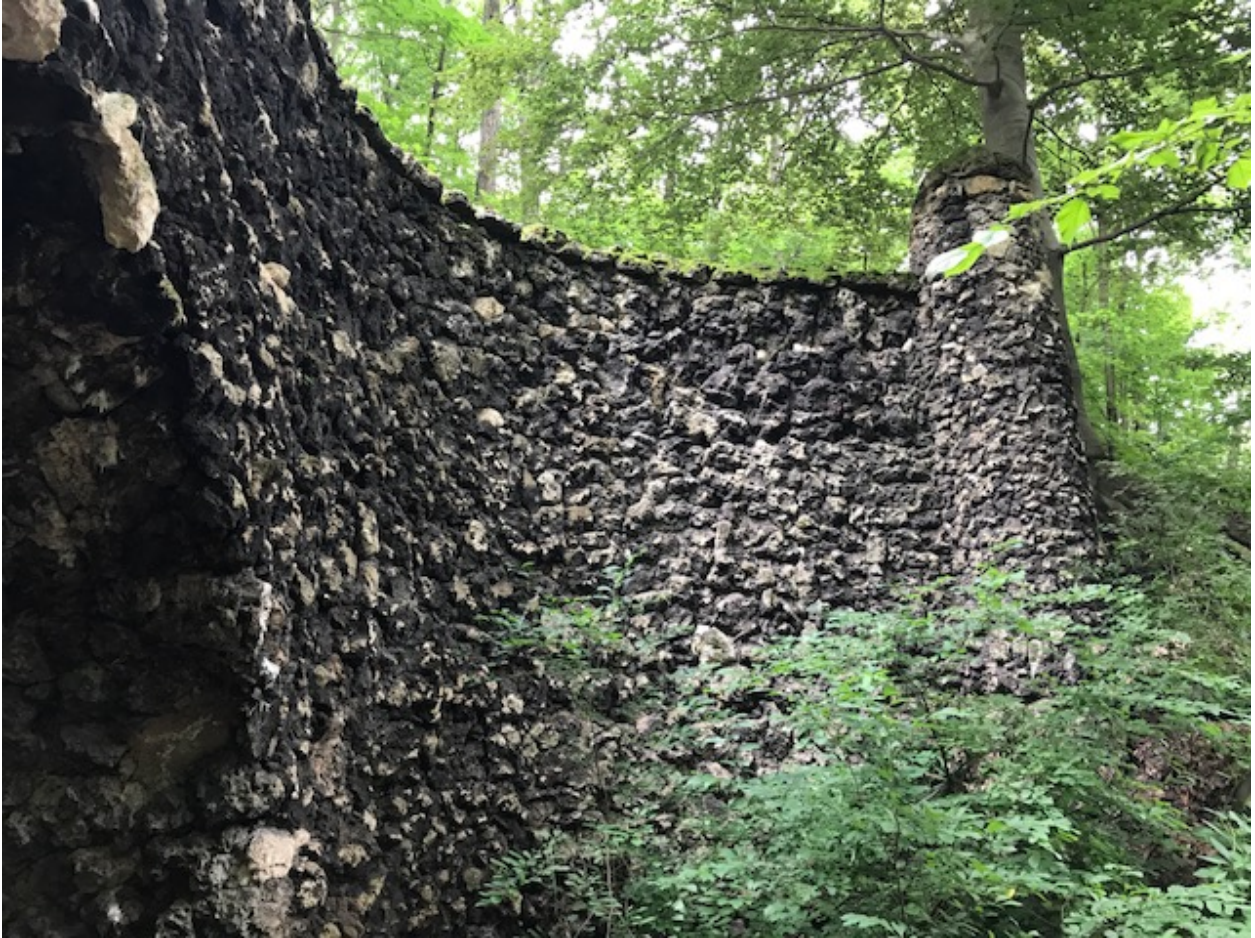
Photo. 3. Tufa Bridge II (Elliptical Arch) , Schenley Park, June 2, 2017. Source: Matthew W.C. Falcone.
