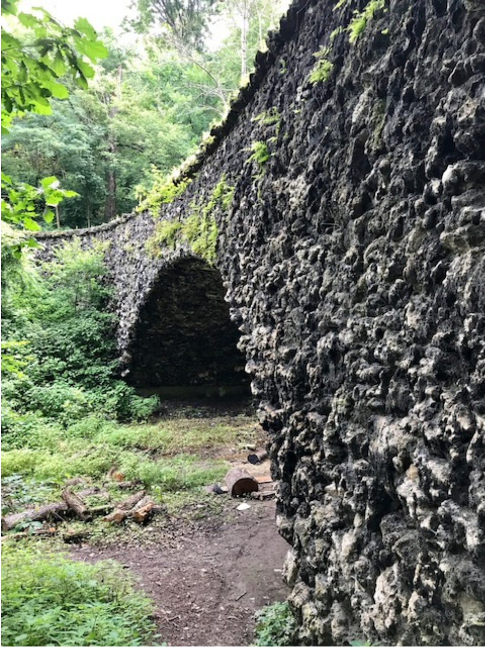
Photo. 2. Tufa Bridge II (Elliptical Arch) , Schenley Park, June 2, 2017. Source: Matthew W.C. Falcone.
